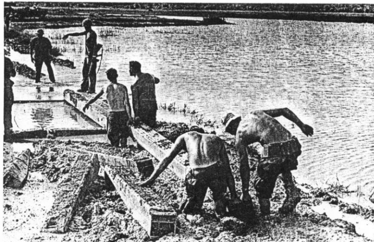
The "White Lions" are probably beginning to wonder if there is a dry place in Vietnam as they start digging and carrying the sections of metal bridge bulk out of the mud.
