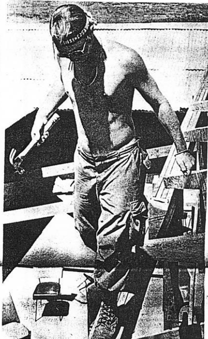
CHU LAI , (23d Inf. Div. IO)—Specialist Four Tim Vincent (San Diego, Calif.) walks a beam on the roof of the Enlisted Men's Club here. Vincent and other personnel from the 23d Infantry Division (Americal) Repair and Utilities division were doing the work project on the EM Club, reusing wood and tin from torn down building in the Americal area. (U.S. Army Photo by Sp/4 Jimmy J. Stallings)
