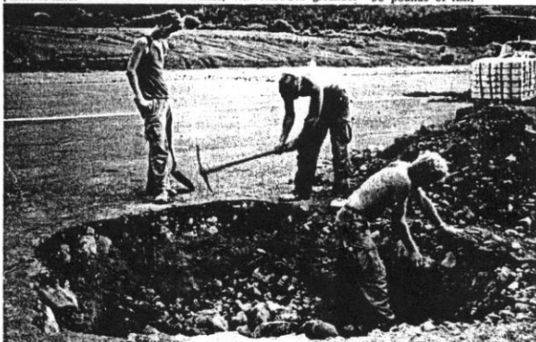
Working under the blazing sun at Kham Duc, these engineers repair the holes in the runway after enemy booby traps were dug out. The Kham Duc runway was recently reoccupied by the Division after its abandonment in 1968. (Photo by PFC Guy Winkler)
