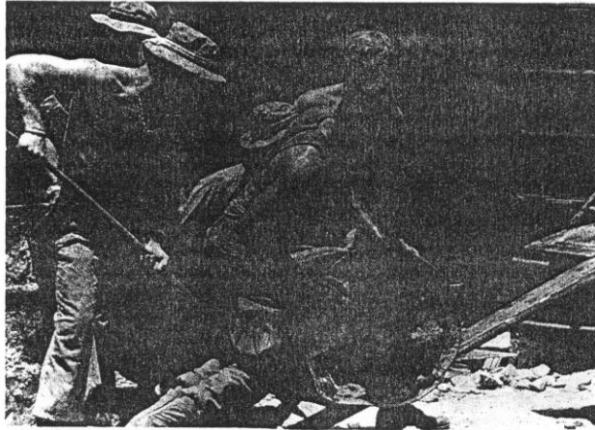
A work party (why they call it a party, we're not sure) at FSB Dottie is trying to coax a 55 gallon drum full of dirt onto a truck. These "Jungle Warriors" of the 11th Infantry Brigade were rebuilding the blast walls around the Brigade TOC. (U.S. ARMY PHOTO BY CPT JOHN J. HOLLINGSWORTH)
