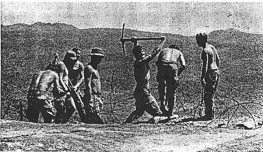
ABOVE: "Look out below", as the roof supports for one of San Juan's numerous bunkers is toppled from its roost. These men are part of 4/21st Bn., whose job it was to remove part of the FSB in preparation for the ARVN's taking over the remaining half.
