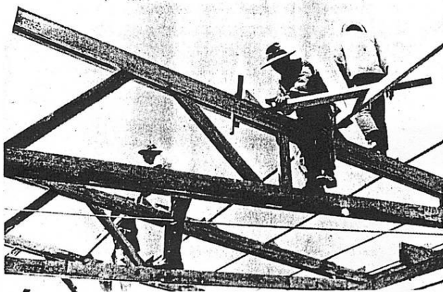
Four Korean workers put finishing touches on the roof supports for the Officers Club roof. The roof, finished with tin, replaced the thatched roof which blew off during a May typhoon. (U.S. Army Photo by Sp/4 Ron Cyderman)
