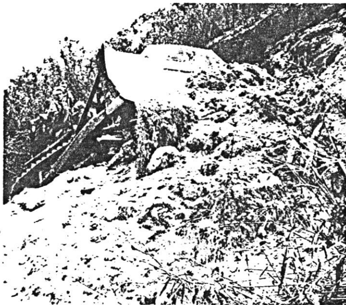
PERCHED ATOP THEIR BULLDOZER, 26th Engr. soldiers move massive mounds of earth in clearing a road to the Tra Bong CIDG camp. Security was provided by A Co., 1-52 Inf., 198th Bde. (Photo by SP4 Mike Friedman, 26th Engr. Bn.)
