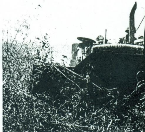
The big blade of a D-7 bulldozer pushes brush and trees before it as it is involved in a land clearing operation around the village. It was supplied by the 26th Engineer Battalion.
