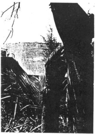
A dozer heads for the larger tree. The dozer was by Headquarters Platoon, Bravo Company of the
