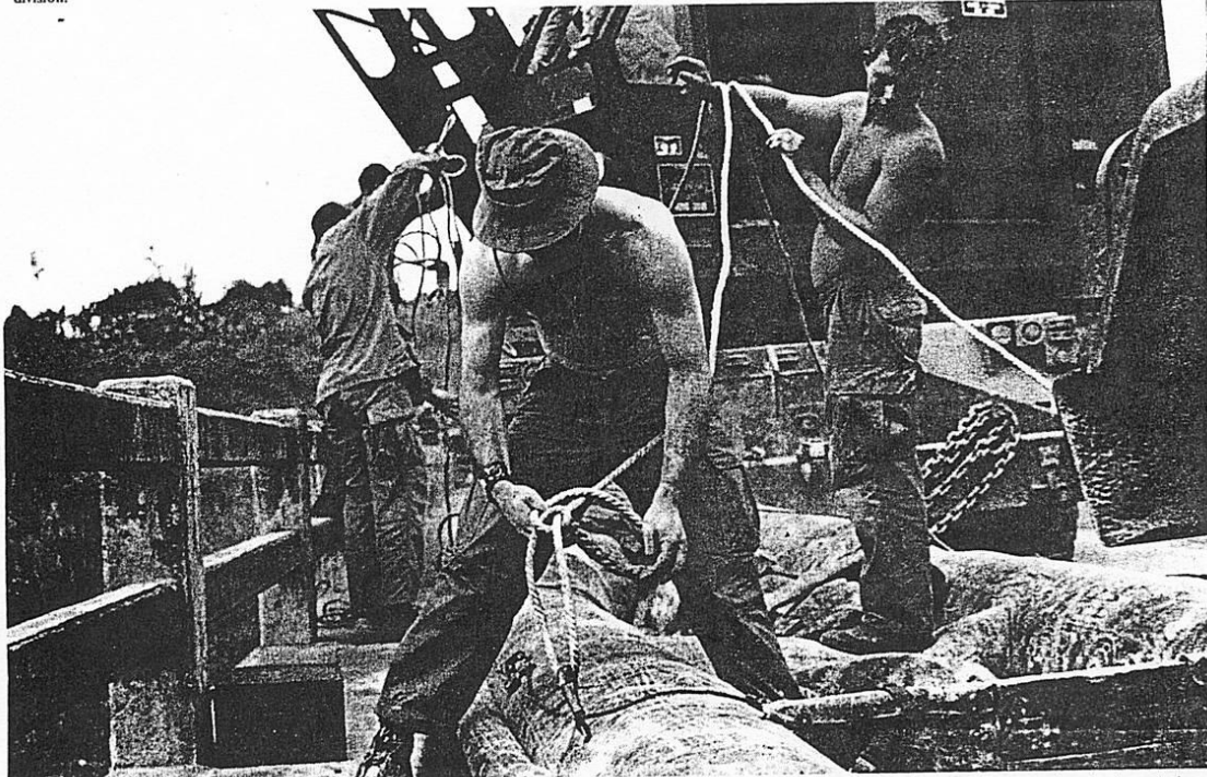
Engineers prepare to hoist a 15 man assault craft over the side of the Quang Ngai Bridge. The craft was employed in assessing mine damage to the supporting piles beneath the 300 foot structure.
