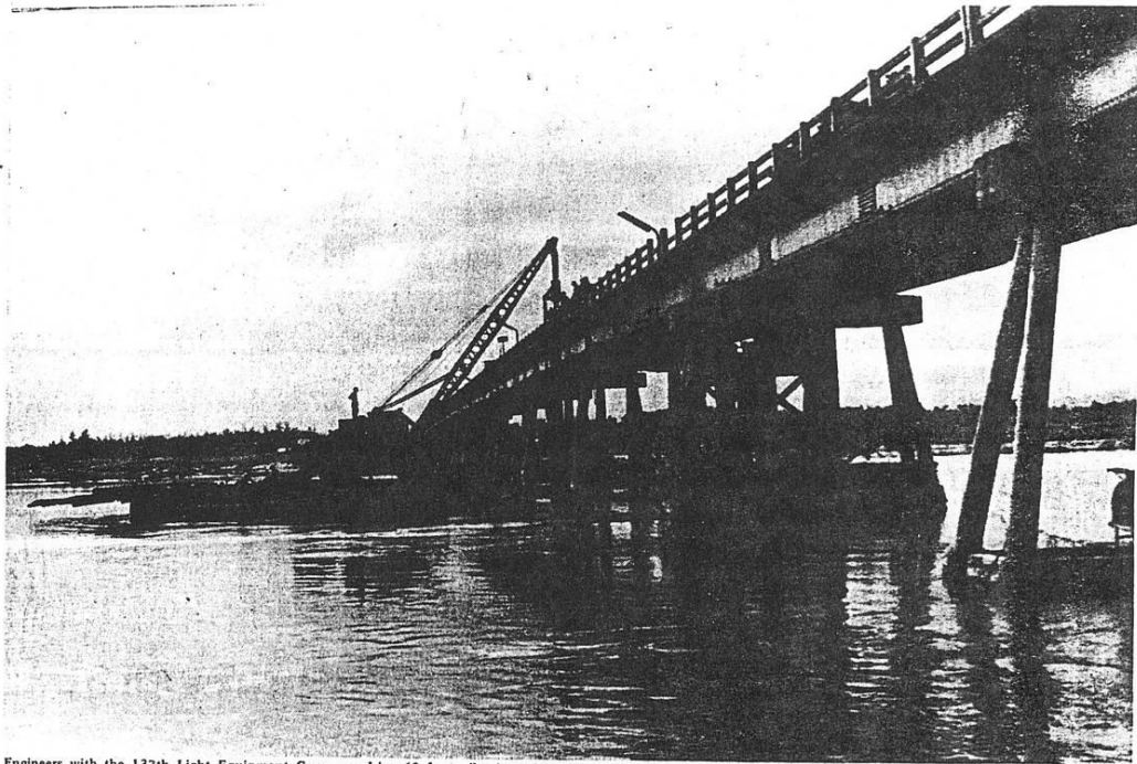
Engineers with the 137th Light Equipment Company drive 60 foot piles into the Song Tra Khuc River, near Quang Ngai. The bridge damaged by a floating mine is being reinforced through the joint effort of Company E, 26th Engineers; Company B, 39th Engineers, and the 137th Light Equipment Company.
