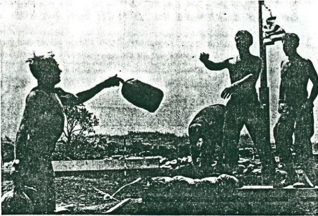
WITH A HEAVE, 198th Inf. Bde. soldiers add another sandbag to a bunker at Fire Support Base Minuteman, the new forward LZ of the 5th Bn., 46th Inf. Minuteman is the first American fire base in the heart of the Batangan Peninsula, a former Communist stronghold for 20 years, 15 miles south of Chu Lal. The fire base—constructed by D Co., 5th Bn., 46th Inf. and a platoon of B Co., 26th Engrs.—is expected to aid in the pacification of the peninsula. (Photo by SP4 John Hollenhorst, 198th Inf. Bde.)
