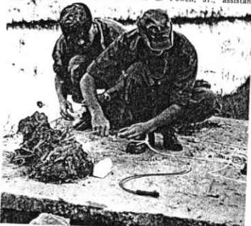
Two demilitarized men assigned to the 26th Engineer Bn. carefully place charges of high explosive on the surface of a concrete slab serving as a footbridge on the old Mo Duc Path. When the charges were detonated, the concrete slab and rails were destroyed, but the abutments of the bridge were untouched, as planned.
