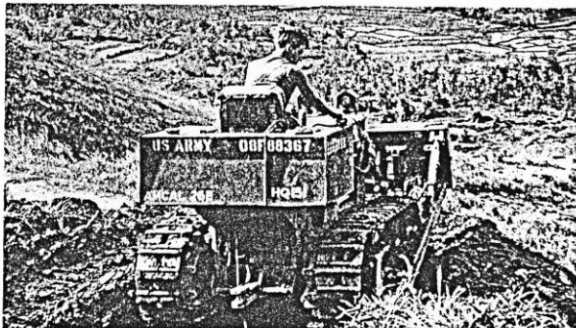
BUILDING AN INTERSTATE FREEWAY? Not really. This member of the 26th Engr. Bn., is leveling out a gun position on LZ Siberia for C Btry 3rd Arty. Since they are in the field a great deal engineers play a dual role, having to be proficient at being both infantrymen and combat engineers. (Photo By SP5 M. L. Hoskinson, Americal IO)
