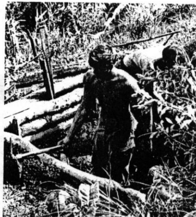
Men of Company A, 4th Battalion, 31st Infantry of the 196th Brigade know the importance of a good foxhole. These soldiers are building their new home on LZ Melon. (Photo by SP4 Jim Logue)
